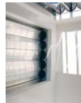
Mixing box with dampers
